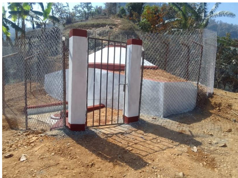
Reservoir tank of Musle Drinking Water Schemes of Manahari-8, Musle, Makawanpur
